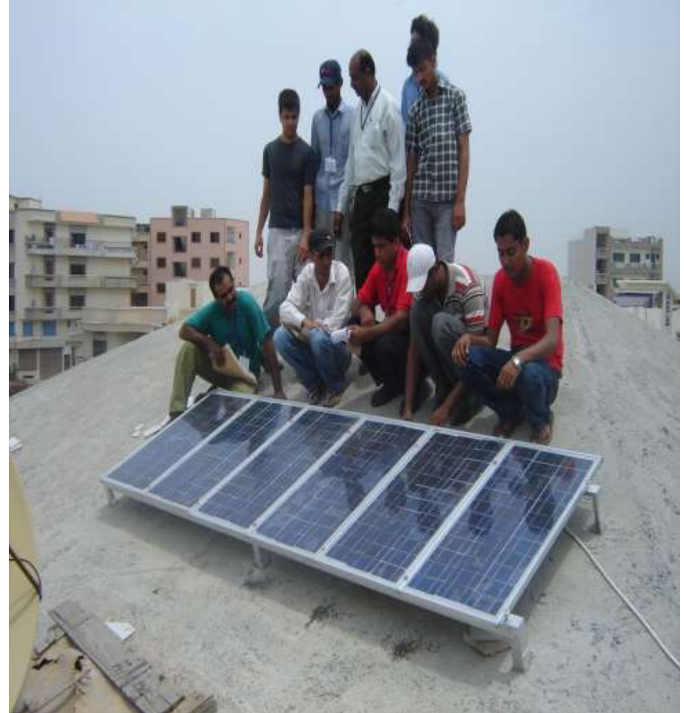
PV array (6X60W) installed
